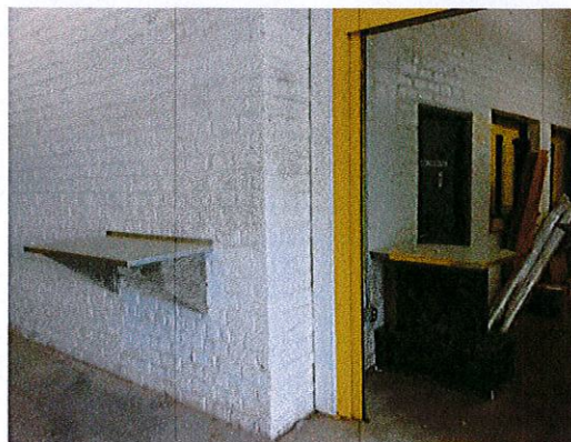
Photo 5: The counter (likely for condiments) across from the concession stands currently creates a protruding hazard.
