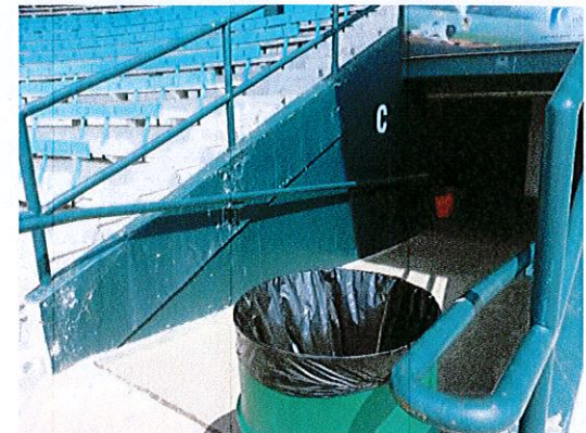
Photo 3: Replace the handrails on the ramps leading to spectator seating with a style that has a 1 1/4"-1 1/2" diameter (currently 3").
