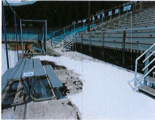
Photo 7: Wheelchair positions have been provided on the wood platform in front of the open metal bleacher system.
