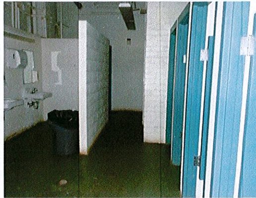
Photo 8: The multi-fixture toilet rooms do not currently provide any features of accessibility. Post signs directing to the single-user accessible toilet rooms.
