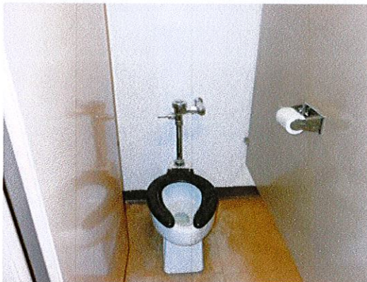
Photo 4: The toilet room does not currently provide any features of accessibility.
