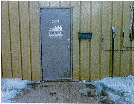
Photo 1: View of main entry. Replace the knob with a style that does not require grasping, pinching or twisting to operate (such as a lever).
