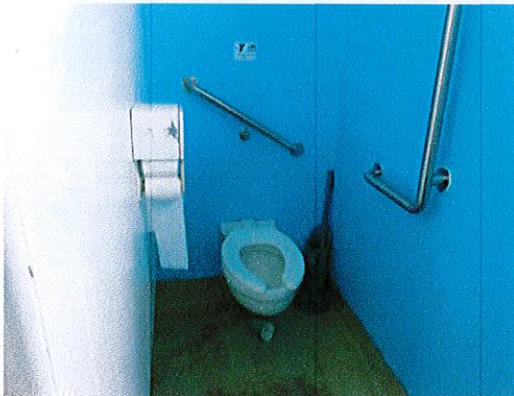
Photo 5: The toilet rooms are not currently accessible (grab bars have been installed but they are not the correct configuration and the stall is too narrow).
