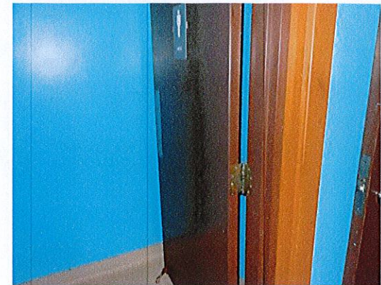
Photo 3: Maneuvering clearance is not currently provided at the toilet room entry doors.
