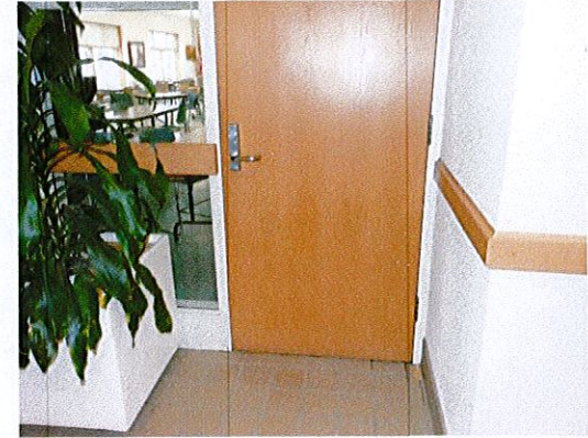
Photo 3: Relocate the planter that currently obstructs the pull side clearance to the small meeting room (103).
