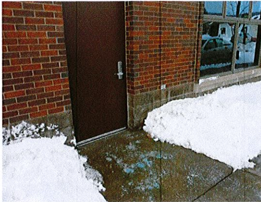
Photo 2: Patch the concrete and expand to provide maneuvering clearance at the exterior door that leads directly into the community room. (This was the primary door used by participants.)
