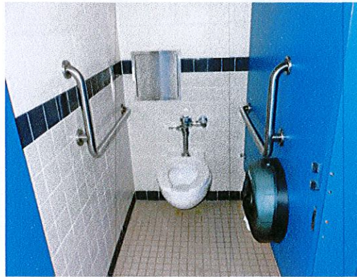
Photo 8: View of toilet room. Typical toilet rooms provide an ambulatory accessible stall, but not a stall with 60" clearance.
