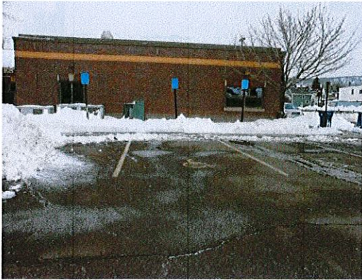
Photo 1: View of parking. Restripe the parking spaces to 8' wide with 8' wide aisle (can be shared between 2 spaces).
