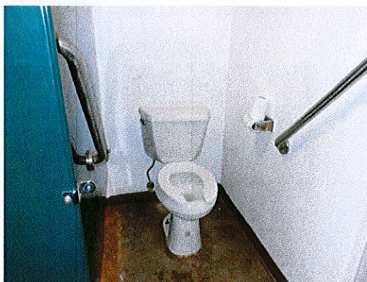
Photo 4: The toilet rooms provide an ambulatory accessible stall, but not a 5' accessible stall.
