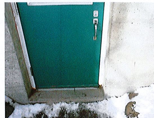
Photo 3: Eliminate the step at the entry to the toilet rooms and replace the thumb-latch style door hardware.
