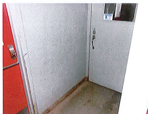
Photo 5: View of vestibule at toilet room entry. The vestibule is too small to provide turning space or maneuvering clearance at any of the doors.
