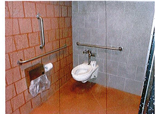
Photo 3: An accessible toilet compartment is provided in the men's and women's toilet rooms. This is a good example of accessibility.
